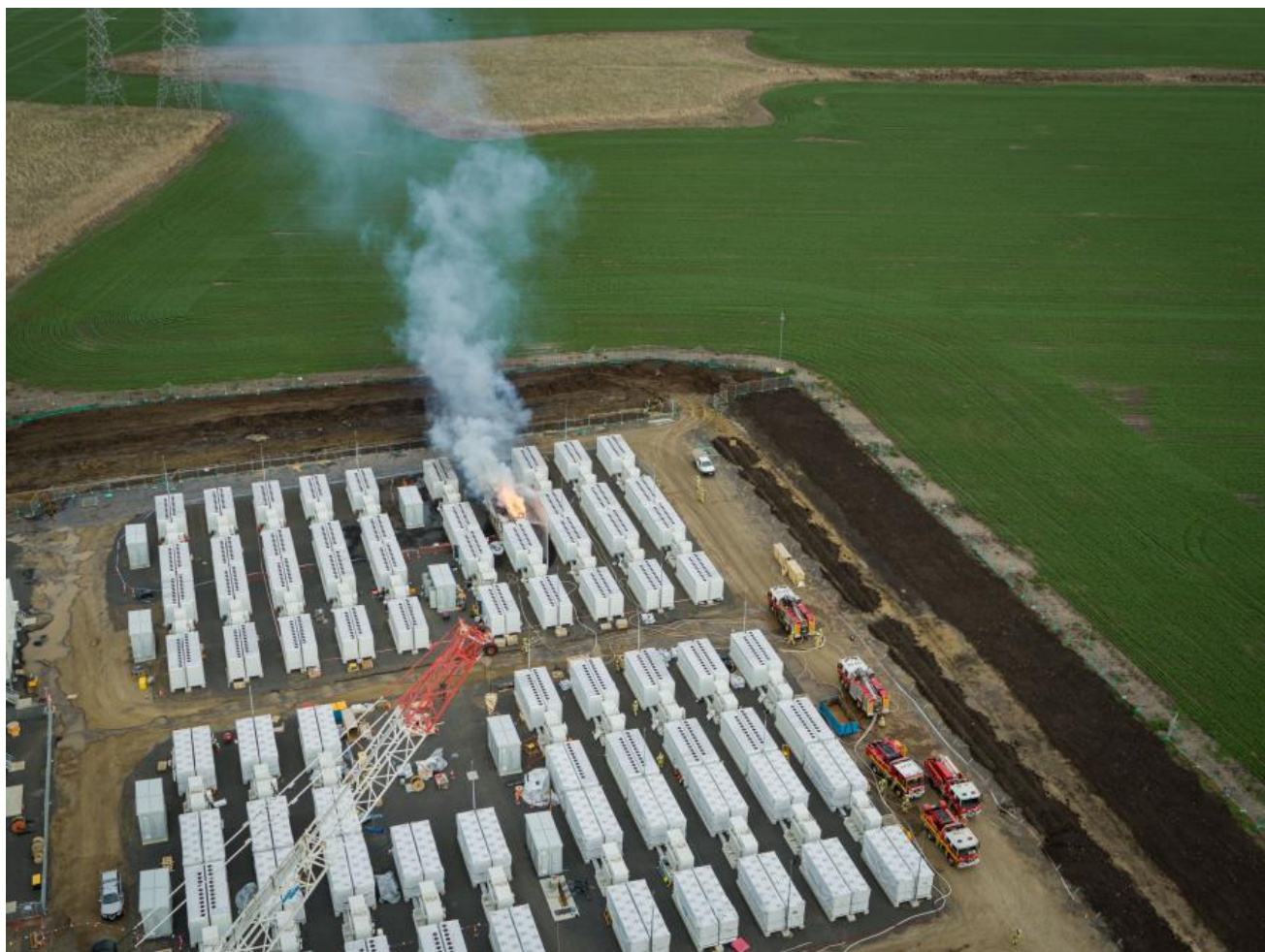
Figure 4 Victoria Big Battery fire incident [47]
